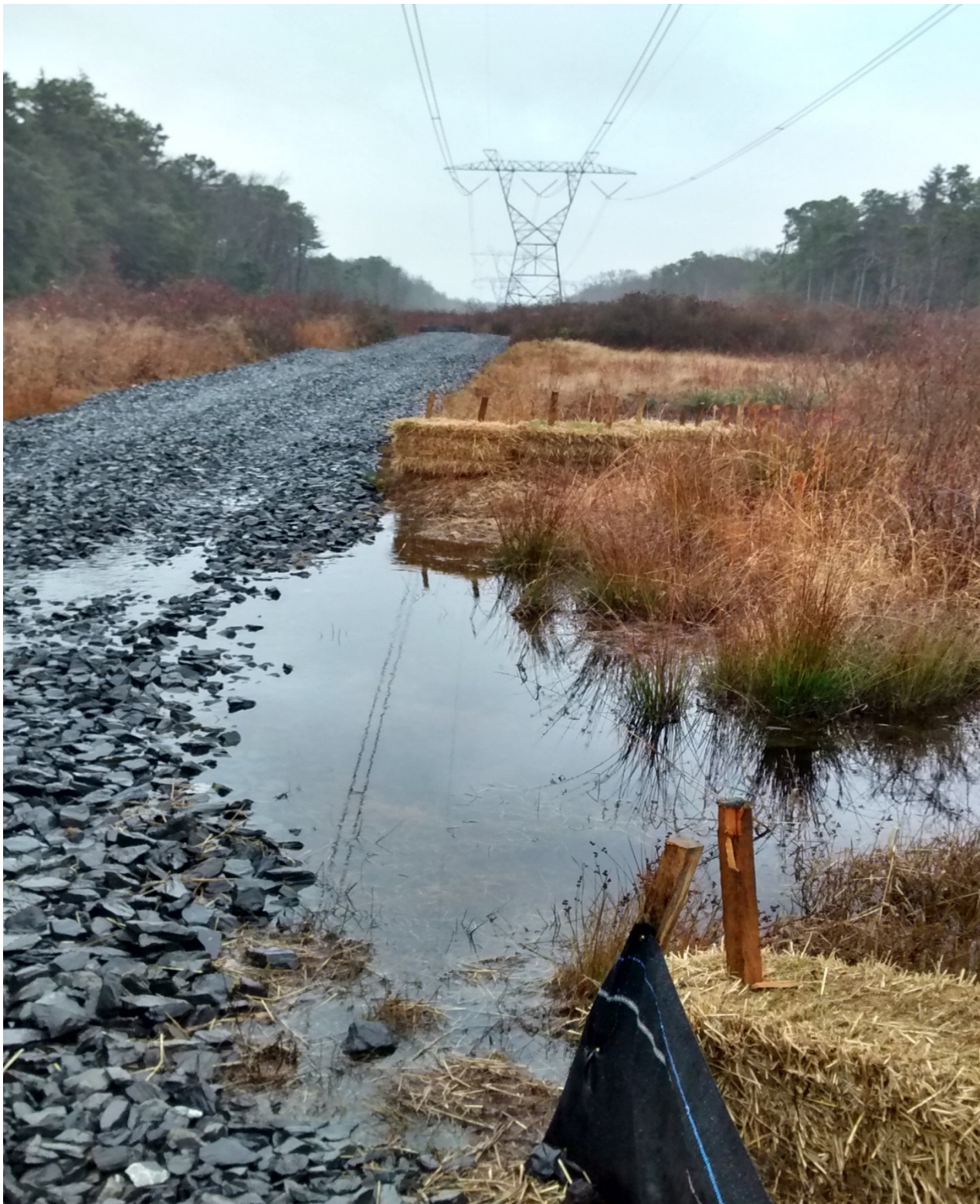
Figure 7: This newly constructed 2015 span access road improvement is beyond the scope of routine maintenance authorized by the ROW Plan. A Pinelands application must be completed for access road improvements beyond routine maintenance.
